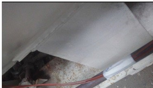
Figure 47. RTD sensor installed on LN 2 fill line
